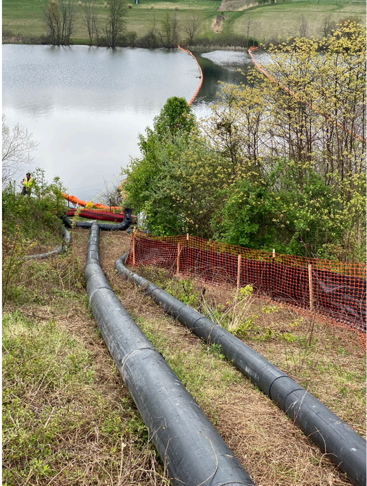
HDPE Conveyance Pipe
