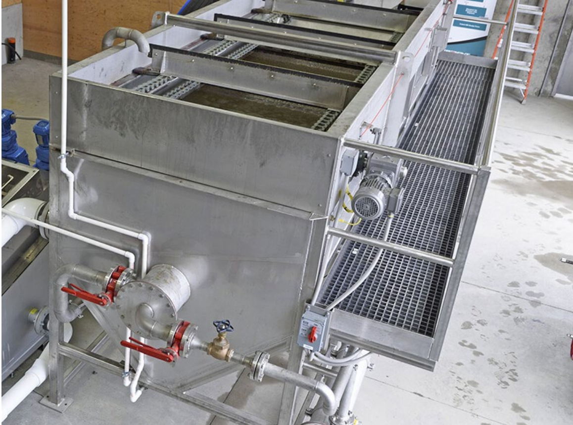
Clarification or Dissolved Air Floatation (DAF) Plant
