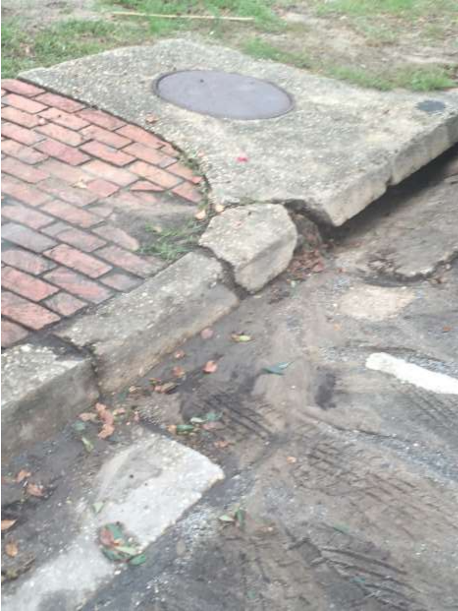
Concrete Damage, Sediment Buildup
