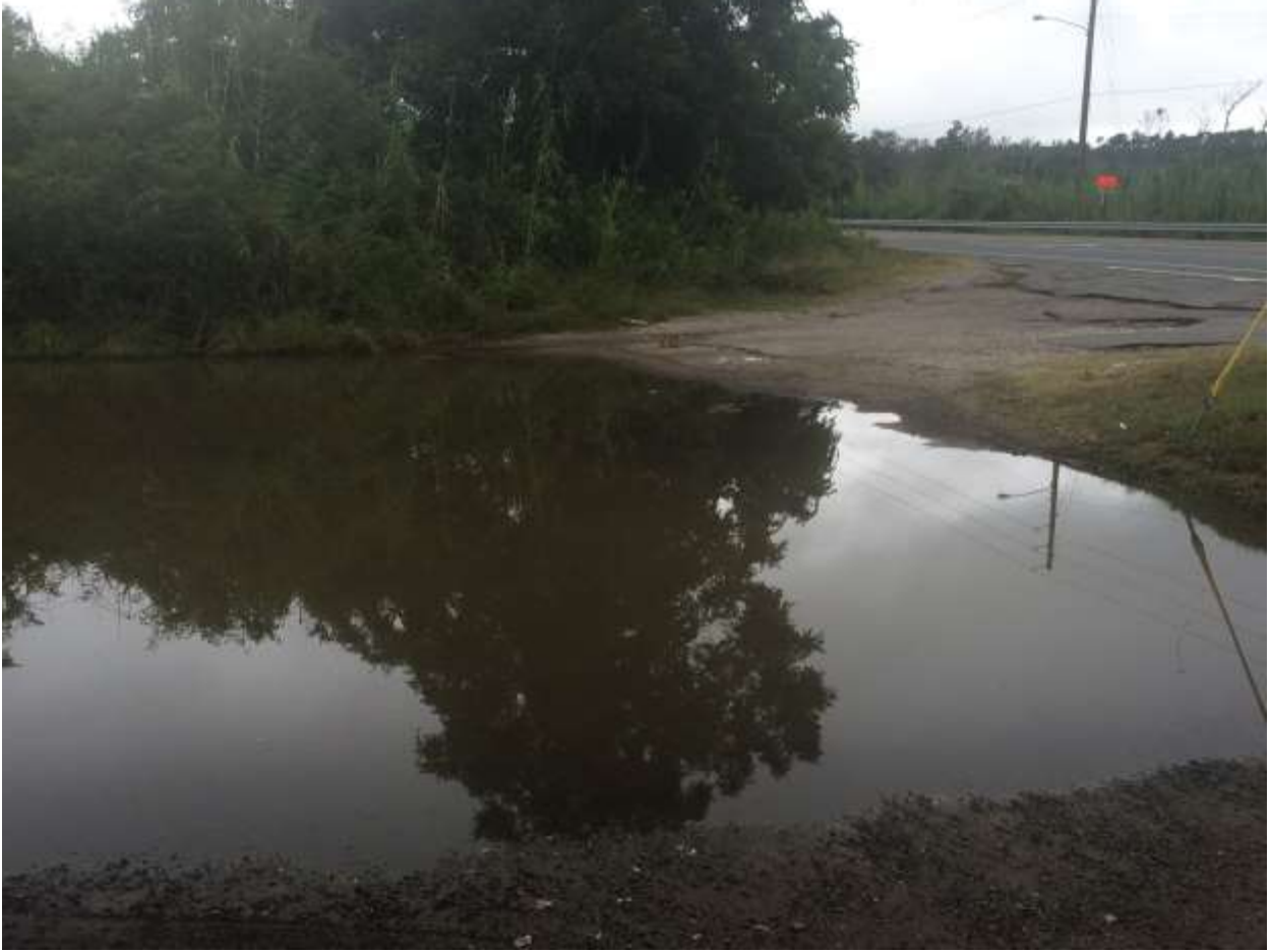
Flooding during 9/29/15 Flooding Event
