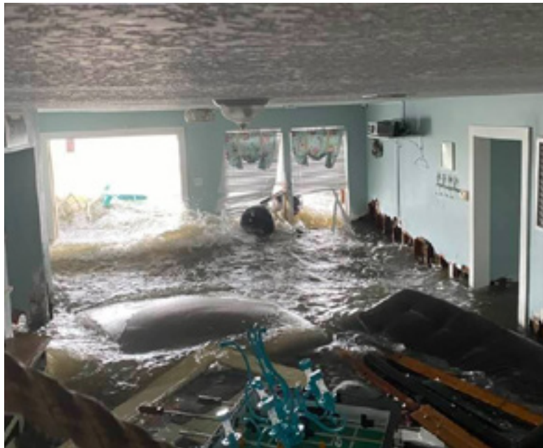
2020 flood damage - Hurricane Sally
