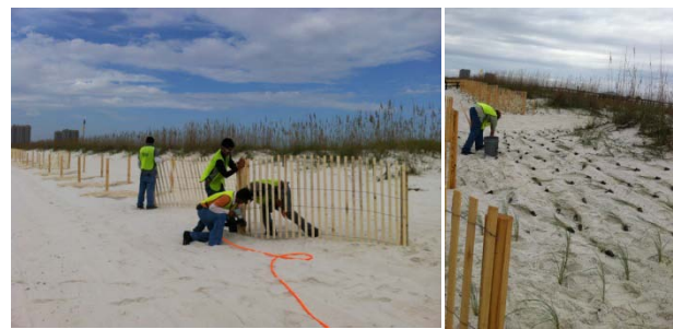
Figure 1: (Left) Contractors adding protective snow fences. (Right) Contractors planting new sea oats.
