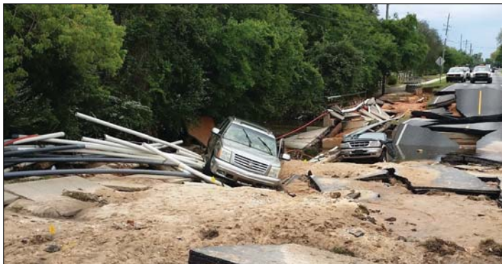
Damage to South Old Corry Road
