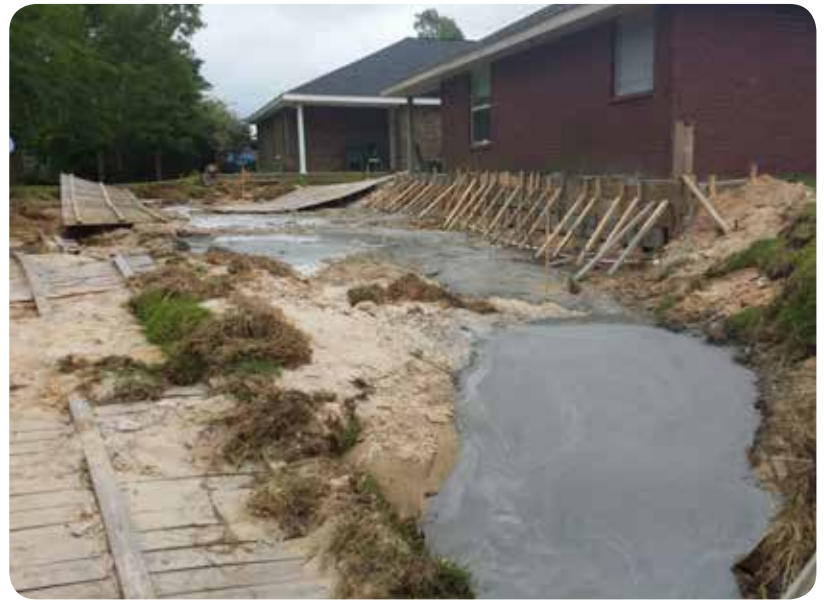
April 2014 flood damage - Newcastle
